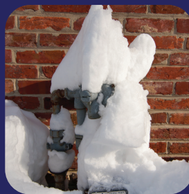
METER WITHOUT SNOW SHELTER
